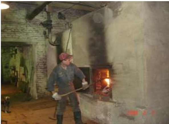
The new economical water heating boiler in the municipal boiler plant in Mikroraion Settlement in Svirsk
