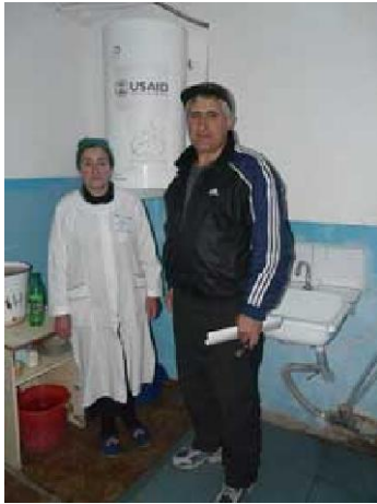
Officials of Agulsky Raion Administration and the staff of the raion hospital located in Tpig Settlement are glad that the hospital now has hot water
